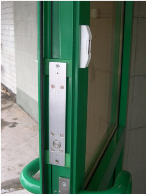
View of the door face with the electromagnetic lock installed inside
