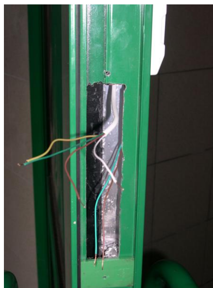
Preparation in the face section of the door mounting hole for the electromagnetic lock
