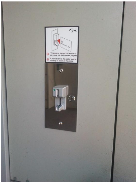
External view of the installed panel with the reader
